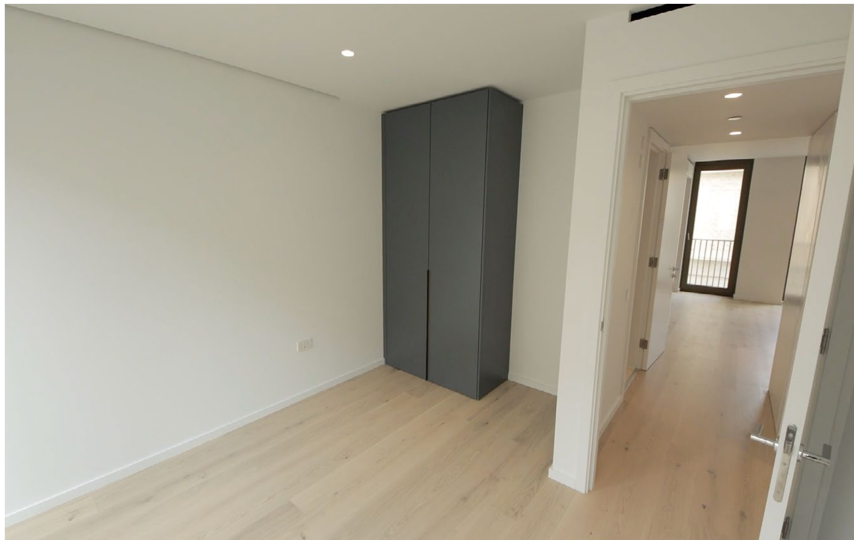
Still image from video footage of second bedroom in apartment 2.6 The Levett Building.
